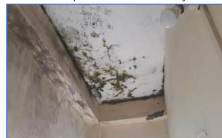
Fungal growth in rooms causing sickness
