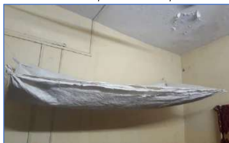
Bedroom covered with plastic sheet
