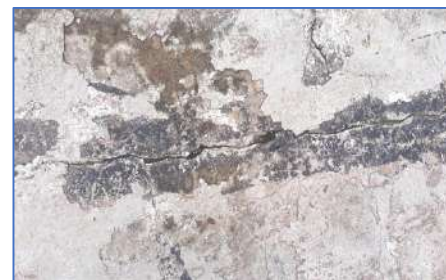
Multiple cracks on the roof
