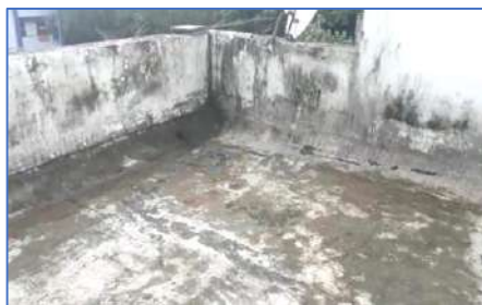
Condition of Leaking Terrace Roof
